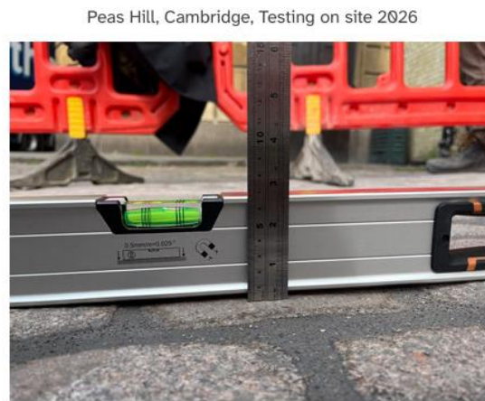
↑ Photo 01: Undulation of 5mm on walkway
