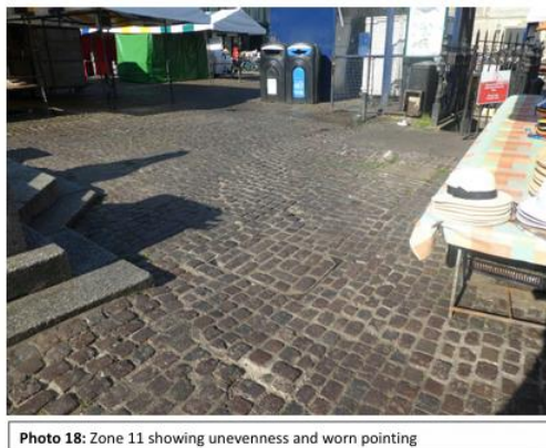
Photo 18: Zone 11 showing unevenness and worn pointing
