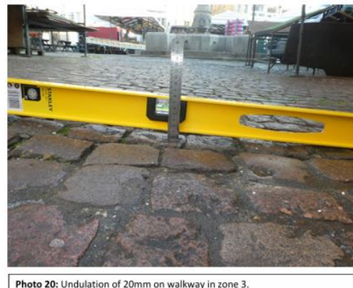
Photo 20: Undulation of 20mm on walkway in zone 3.
