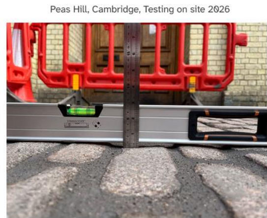
↑ Photo 03: Undulation of 8mm on walkway
